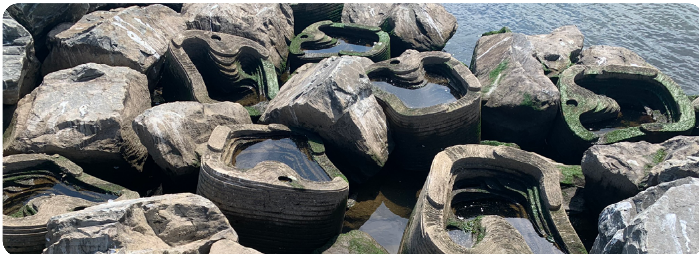
Artificial tide pools provide habitat for marine life in New York Harbor as part of the Living Breakwaters project. Photo: SCAPE. Project designer: SCAPE. Project sponsor: NYS Office of Resilient Homes and Communities
