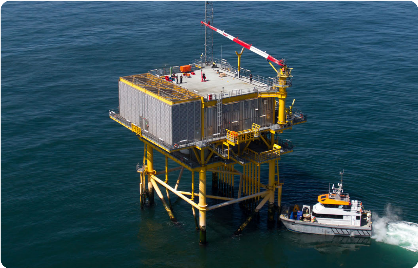
Offshore substations are critical connection points between the grid and offshore renewables.
